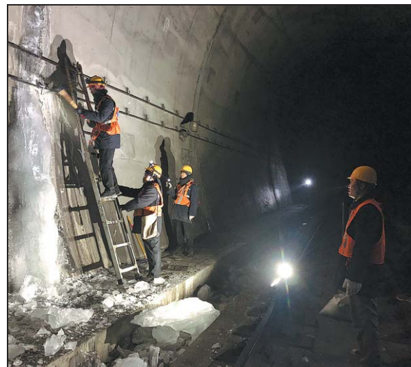
Members of the maintenance squad clear ice on the wall of a tunnel along the Lyuliang section of the Taiyuan-Zhongwei-Yinchuan railway in Shanxi province. SUN RUISENG / CHINA DAILY
