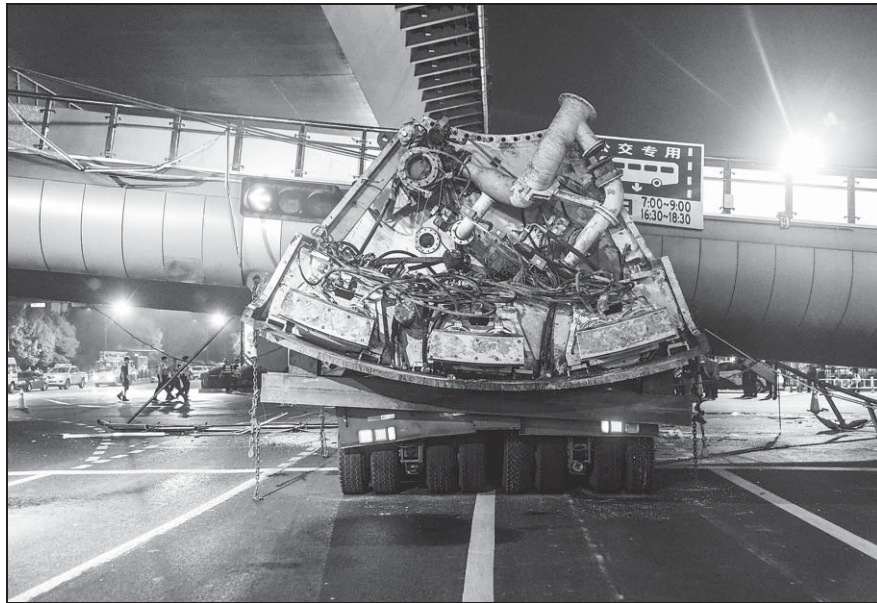
A pedestrian overpass rests on a truck carrying machinery after the truck ran into a pillar holding the walkway up in Hangzhou, Zhejiang province, on Saturday night. No one was injured in the incident. The driver, surnamed Ma, was held by the police. The road reopened on Sunday morning after a cleanup operation. XU KANGPING / FOR CHINA DAILY
